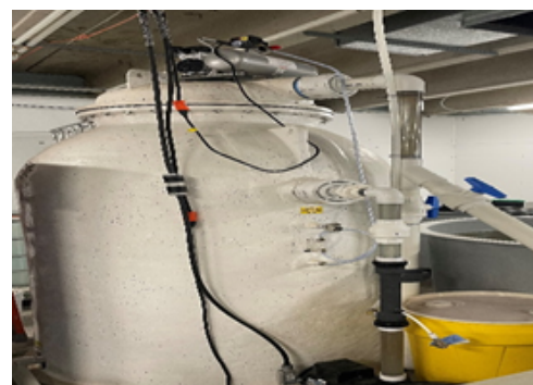
Figure 15: Polygeyser HPPG 25 biofilter.
