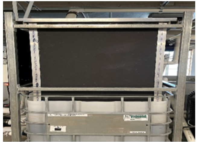
Figure 8: Sideview of the carbon dioxide degassing tower.
