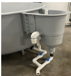
Figure 3: Side drain structure in operation.
