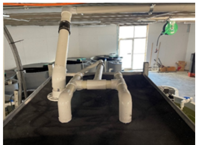
Figure 9: Carbon dioxide degassing tower sprayer manifold and air exhaust vent.
